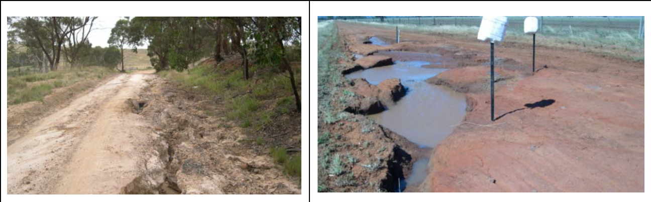
Figure 16: Rain and unpaved (clay) roads do not go together
